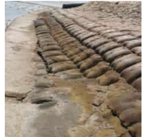
Old damaged protection works
